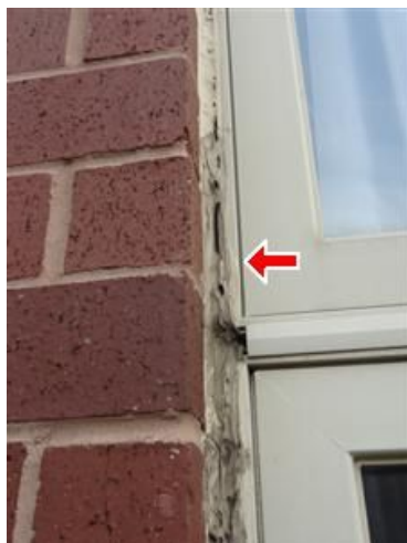
A. Picture 2 Aged and Deteriorated Caulking
