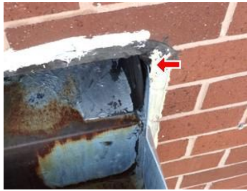
A. Picture 23 Loose Flap of Roofing Membrane At Scupper Opening
