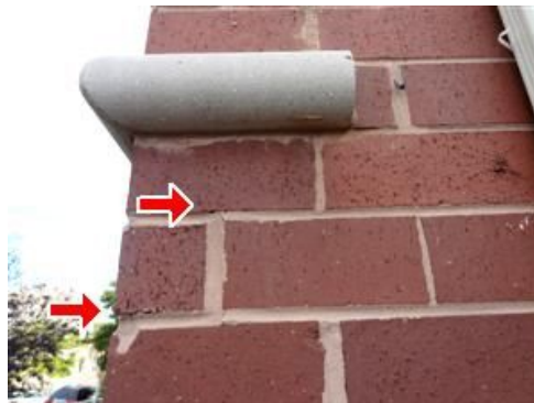
A. Picture 13 Substandard Cement Mortar
