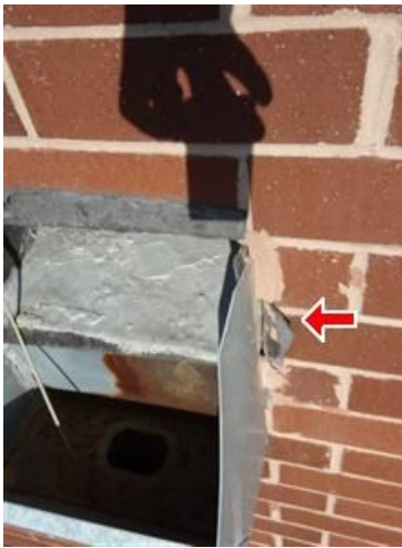
A. Picture 25 Risk for Moisture Penetration at Scupper
