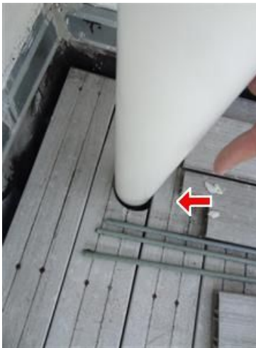
B. Picture 12 Loose Vent Pipe
