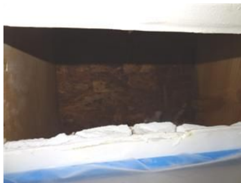
D. Picture 1 Mold-like Substances on Underside of Roof Sheathing
