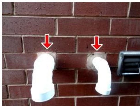
A. Picture 6 Improperly Configured Wall Penetrations
