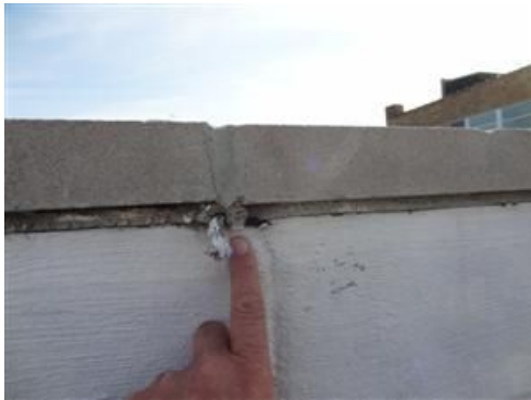
A. Picture 18 Improper Limestone Coping And Flashing Details
