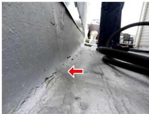
B. Picture 2 Creates That Roofing Material
