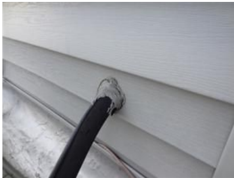
A. Picture 26 Improper Vinyl Siding Penetration
