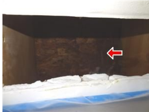
E. Picture 3 Mold Growth at Underside of Roof Sheathing
