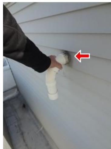
A. Picture 29 Installation of Vinyl Siding Mounting Blocks Recommended e pre-formed vinyl siding mounting blocks that are risk for moisture intrusion. They also allow the siding to amage, sealant failure, etc. Repair by a qualified siding
