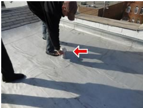
B. Picture 6 Inappropriate Installation
