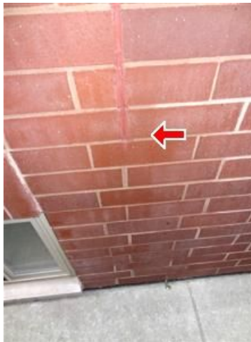
A. Picture 5 Incomplete Movement Joint
