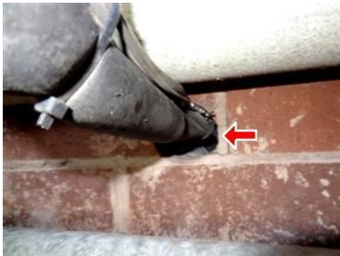
A. Picture 9 Unsealed Air-Conditioning Refrigerant Line Penetration
