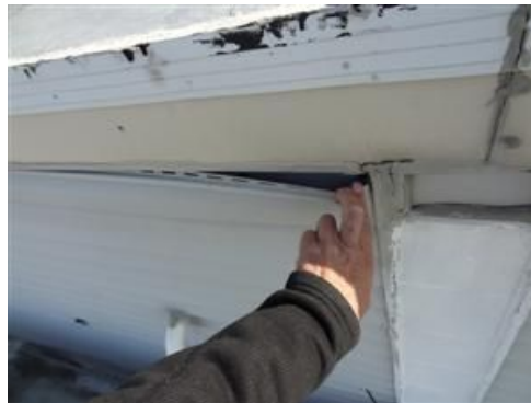
A. Picture 31 Loose Siding
