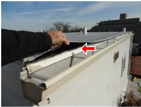
B. Picture 9 Unsealed Roof Membrane
