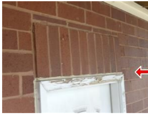
A. Picture 17 Improper Door Installation
