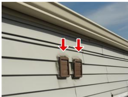
A. Picture 28 Improper Vinyl Siding Penetrations
