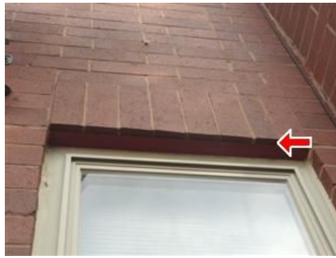
A. Picture 11 Missing Flashing
