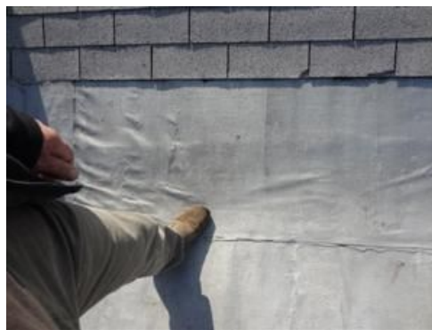
B. Picture 8 Spongy Roof Sheathing
