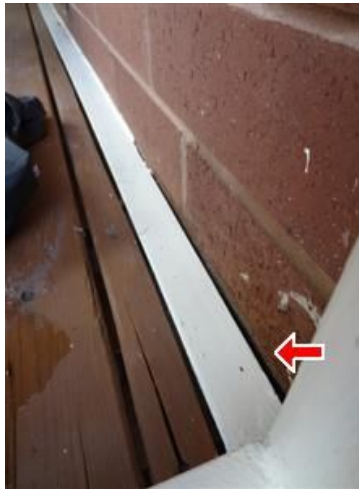
A. Picture 8 Incomplete Sealant Joint
