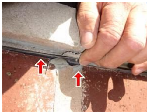
A. Picture 21 Improper Parapet Capping Detail
