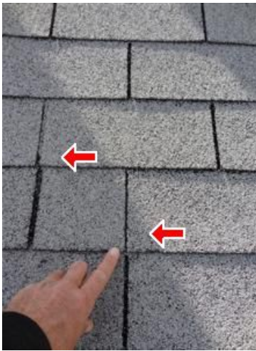
B. Picture 5 Improper Shingle Application
