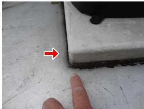
B. Picture 4 Risk for Damage to Roof Covering
