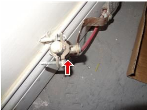
C. Picture 1 Improper Electrical Connection
