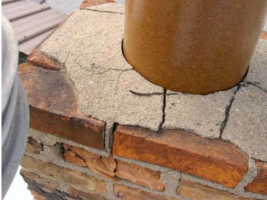
Figure 3 North chimney. Note deterioration of brick & cap
