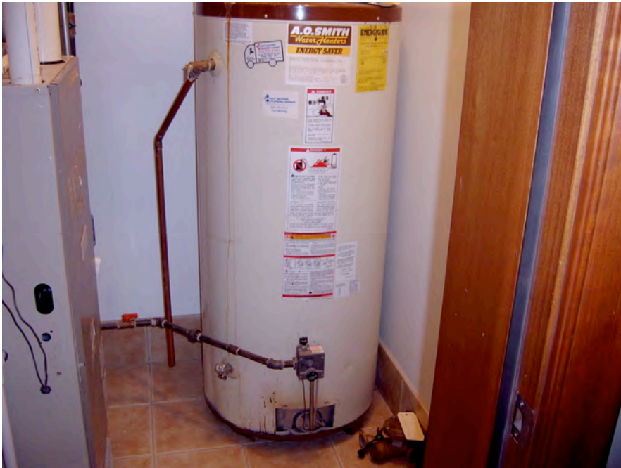
Figure 10 Water heater. Note missing burner cover.
