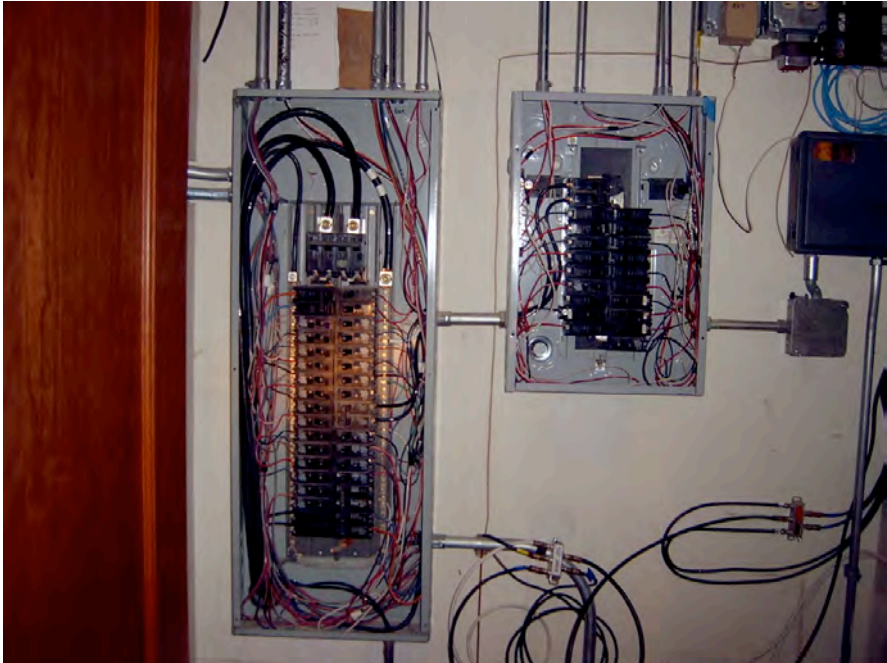
Figure 11 Main electric panels (covers removed for inspection)
