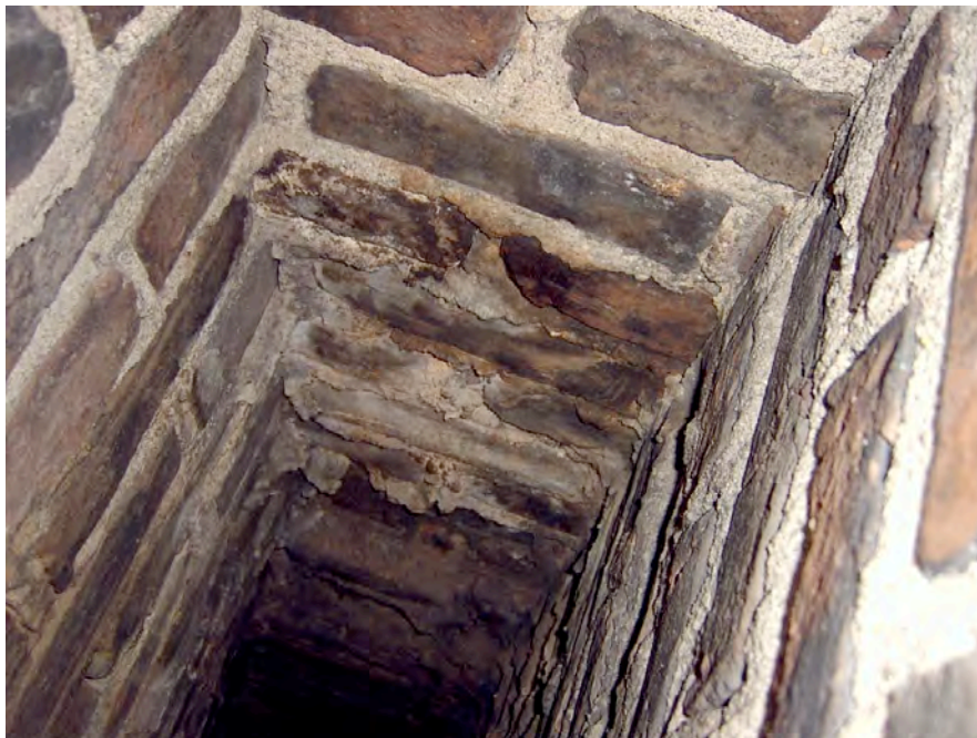
Figure 4 Unlined fireplace chimney
