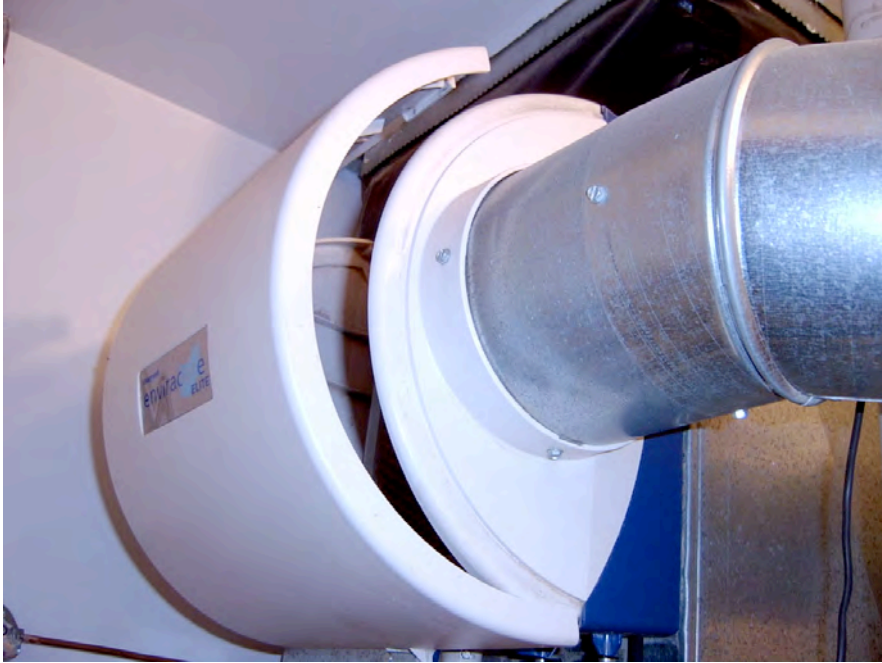
Figure 9 Loose cover on lower humidifier
